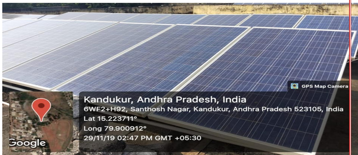
Photograph of solar power panels on the roof top
